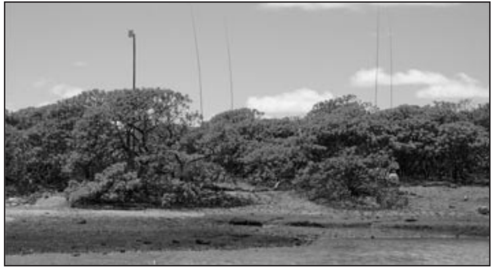
Microwave link antenna on six-meter bamboo pole used for data link between the east and west radio camps. 75M 4-square antenna in the background.
