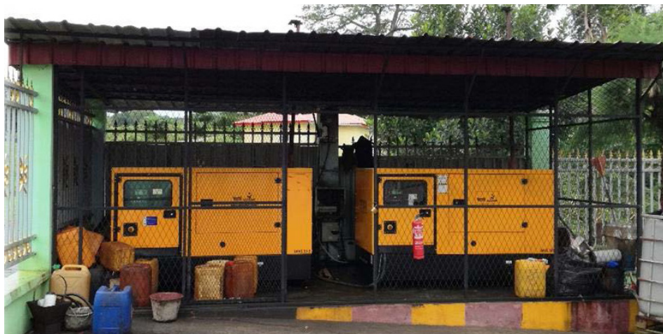
The two 36kW generators.
