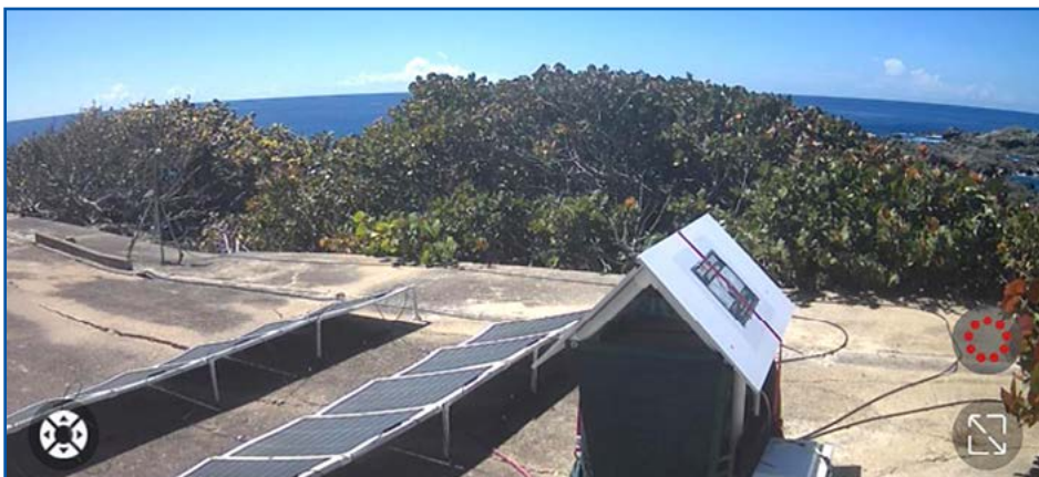
The RDU Unit in its own house with two 2 arrays of solar panels for power.
